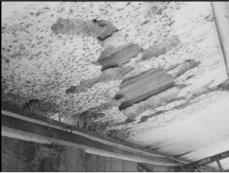
Figure 13.5 - Ceiling insulation damage by mice subsequent to darkling beetle damage.
