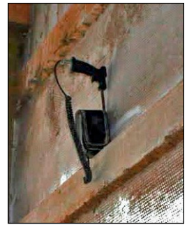
Figure 47. A dedicated, easily accessible thermometer is recommended.
