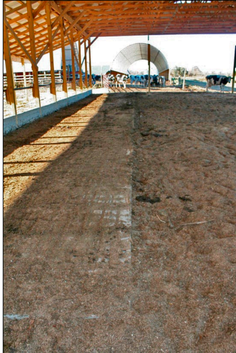
Figure 12. Without a retaining wall or fence separating the pack area from the feed alley, managing moisture in this barn may be challenging.
