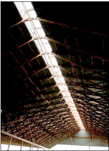
Figure 32. An open ridge vent with an upstand provides maximum air removal with minimal chance of precipitation entering the building.
