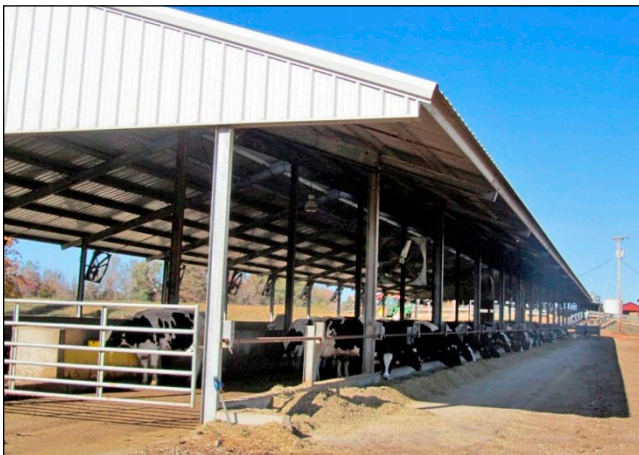
Figure 28. Eave overhangs can help minimize the amount of wind, precipitation, and sunlight entering the barn.
